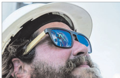
Ryan Fitzpatrick looks at his co-worker Tim O'Gara on a ladder Thursday afternoon as they work on replacing crossing signals at Lisbon Street and East Avenue in Lewiston.
